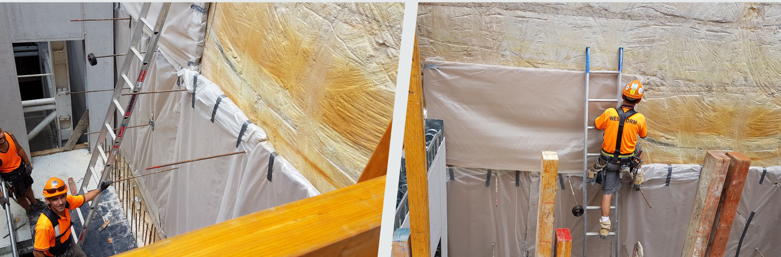
Creating a void between a deep sandstone cutting and adjacent structure - Sydney CBD
